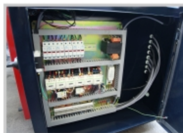
Electrical Cabinet 电器箱
